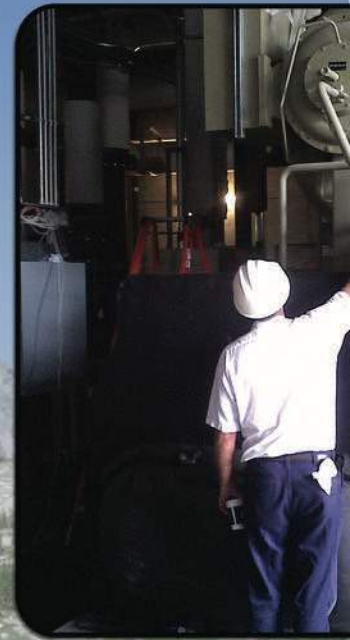
Above: This 2,000 ton system was evacuated from 2,000 microns atmosphere to 1,000 microns in 1 day instead of days with a belt driven pump.
